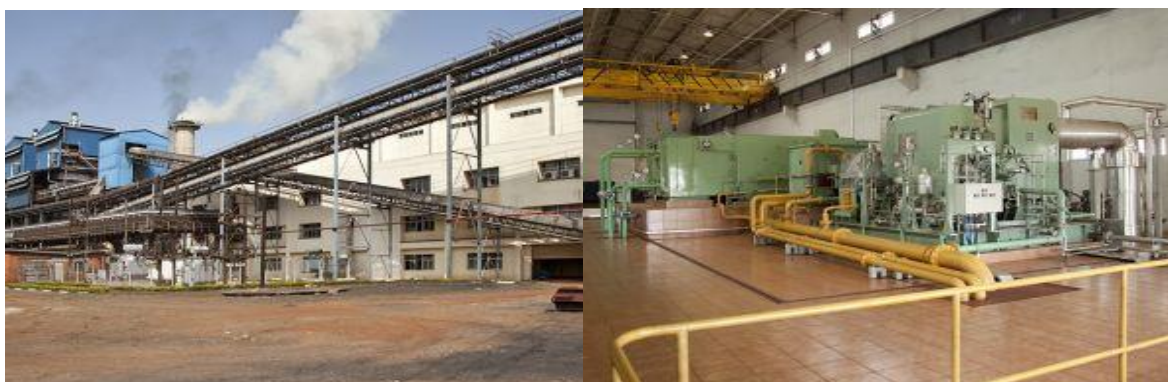
Photos of Kakira Sugar Company's 30MWe Cogeneration Plant, Uganda
